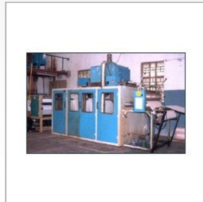
Base Paper (Filter) Impregnation Coating Plant
